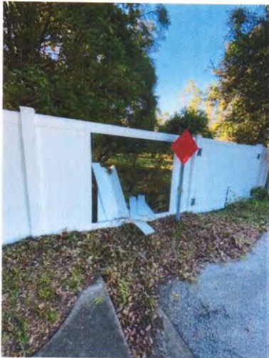
Missing fence panels(Before):
